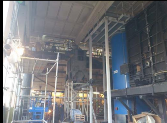
Conversion of a natural gas boiler-house into a biomass boiler in Garliava, Kaunas Region
